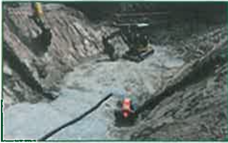
King County Water District No. 90, staff working to repair and improve area infrastructure.
